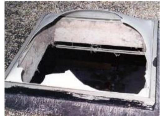
NIOSH FACE Skylight Fatality
