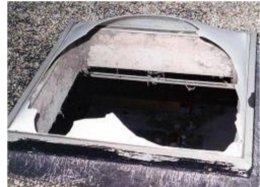
NIOSH FACE Skylight Fatality
